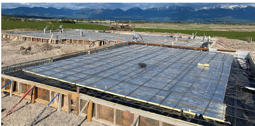
Polyiso insulation installed below slab. Photo courtesy of Malm Construction (Montana) and Big Sky Building Supplies (Montana).
